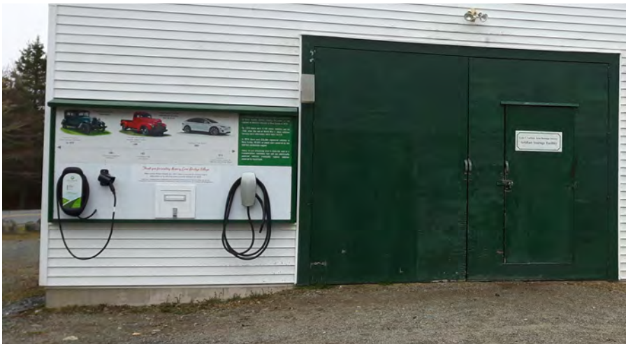
Electric vehicle charger installed on the Artifact Storage Facility (2018)
