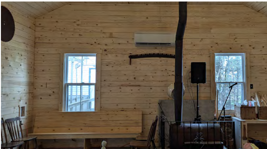
Heatpump installed in the Cookhouse in 2025
